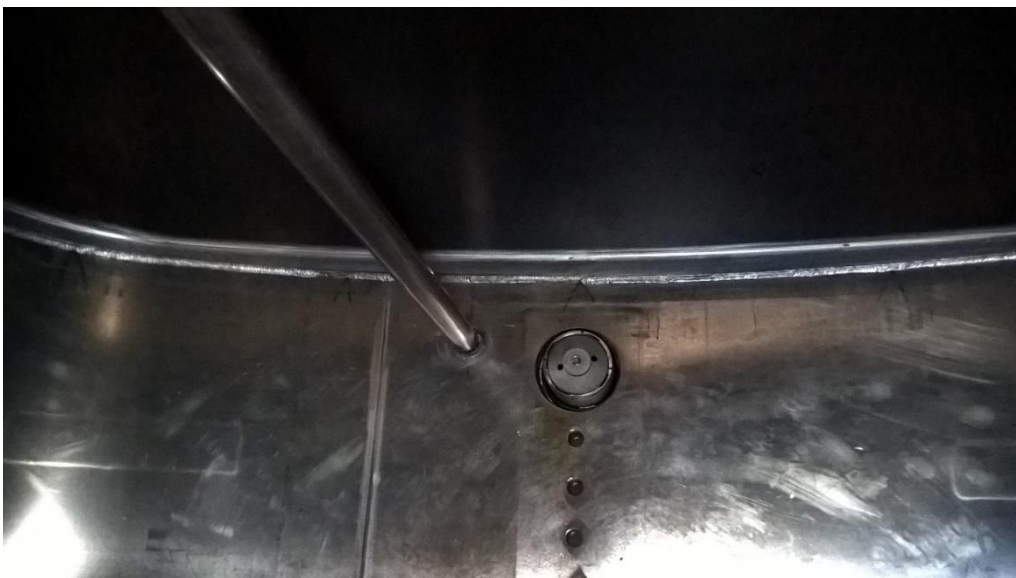
Footvalve within Tank Compartment
